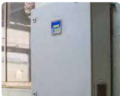
Energy monitoring system implementation
