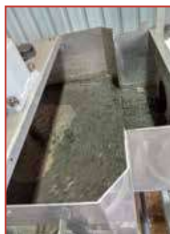
Sludge Mixing Tank
