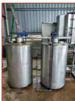
Chemical Mixing and Dosing Unit
